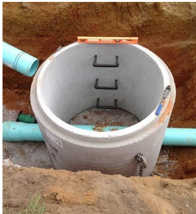
Photo 5: Manhole for gravity Line
