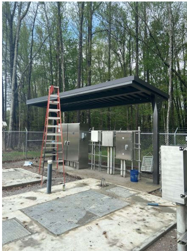
Photo 2: Gadsden pump station
