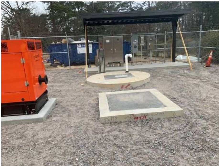
Photo 4: Trotter pump station
