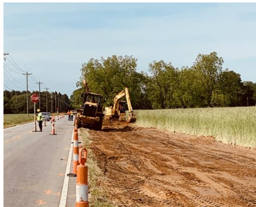
Photo 5: Flagger directing traffic due to lane closure
