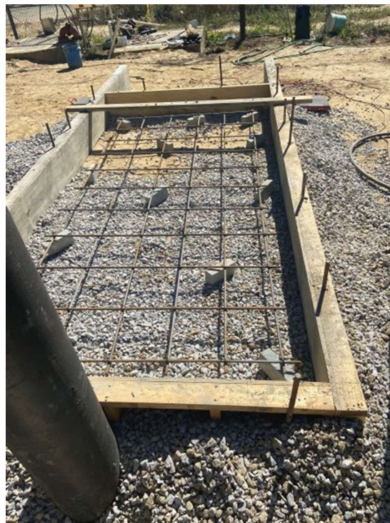
Photo 1: By-pass pump pad
