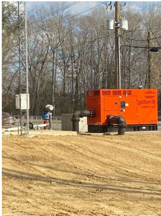
Photo 1: Garners Ferry pump station
