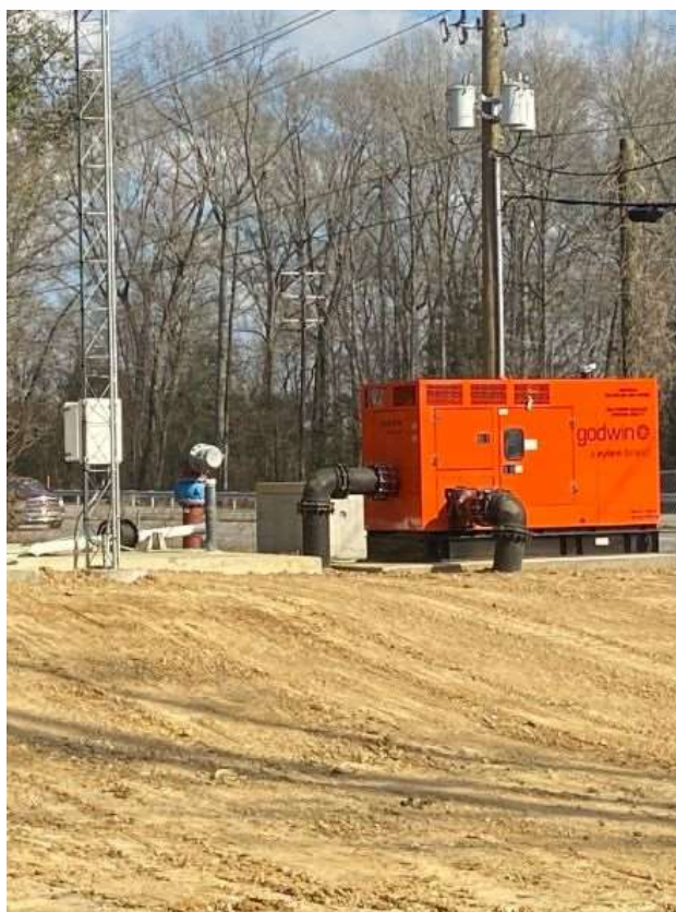
Photo 1: Garners Ferry pump station
