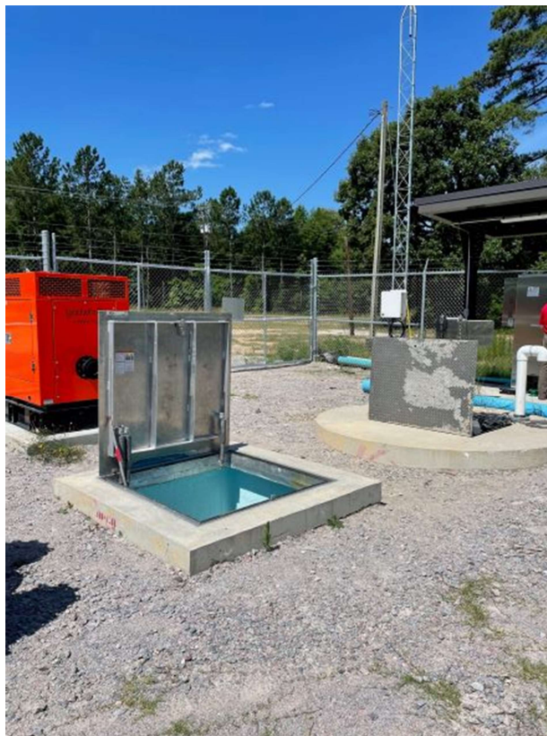
Photo 4: Trotter pump station
