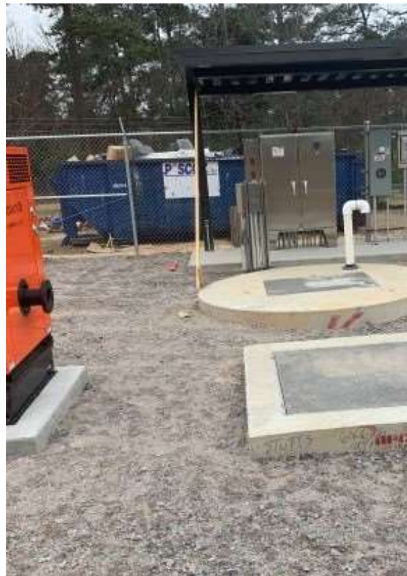
Photo 4: Trotter pump station
