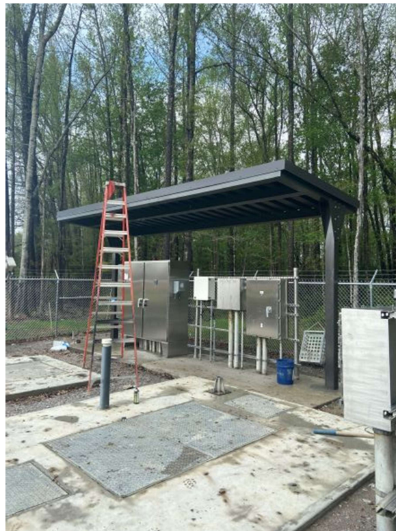
Photo 2: Gadsden pump station
