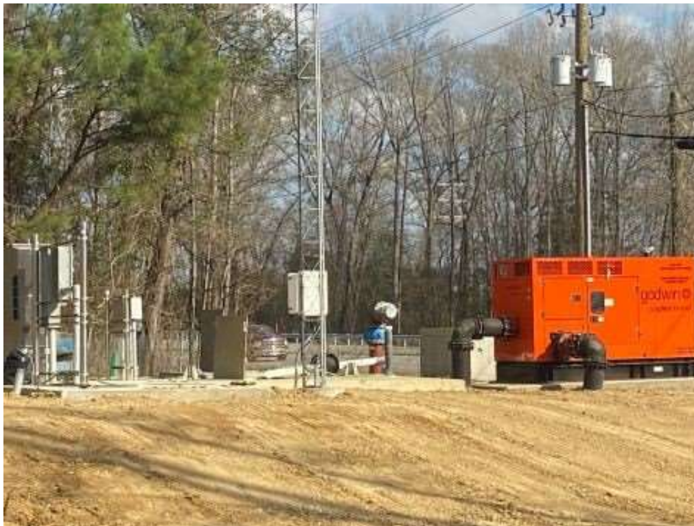
Photo 1: Garners Ferry Pump station
